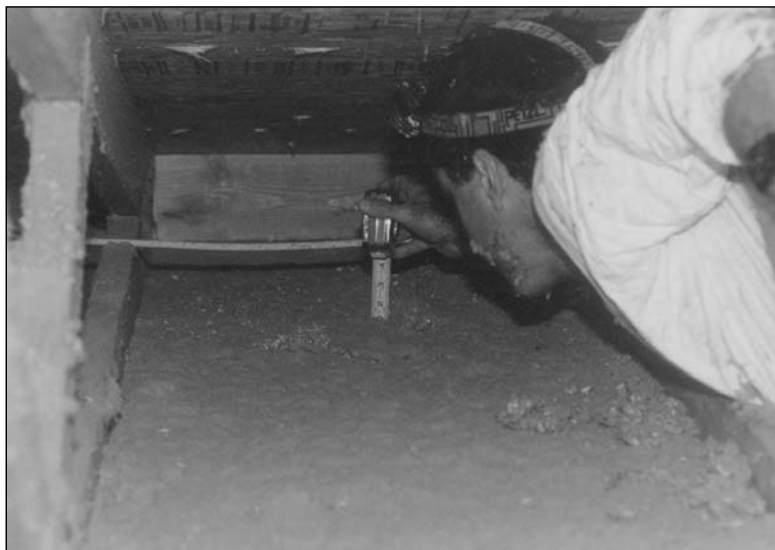
To identify shorting of attic insulation, nothing takes the place of an actual inspection.
